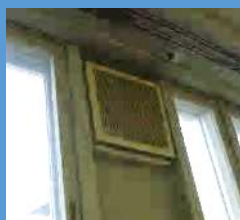
窓設置の換気扇
